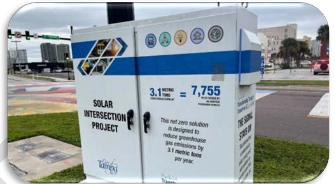
Figure 82. Solar sidewalk battery pack to store energy for power outage events.
