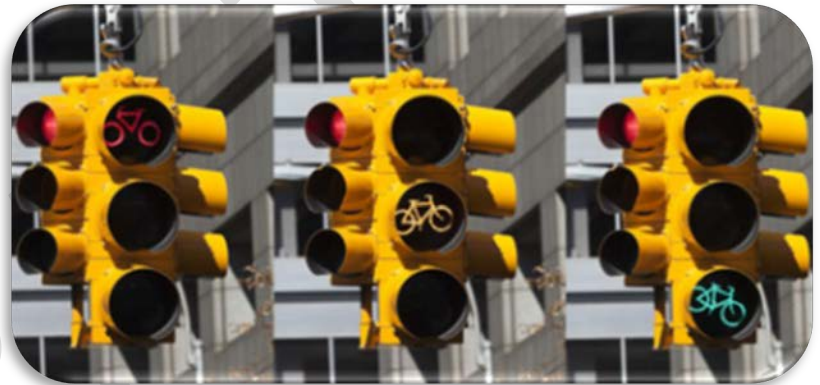
Figure 100. Bicycle traffic signals can be equipped with sensors for data collection .
