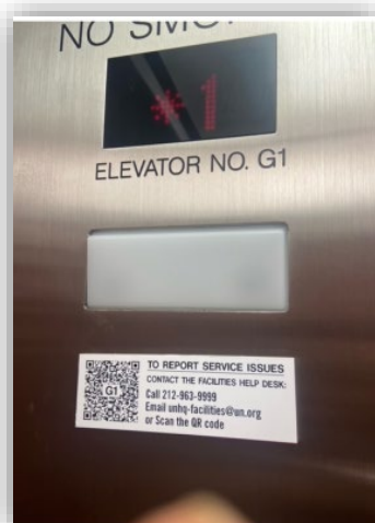
Figure 29. Elevator with QR code.
